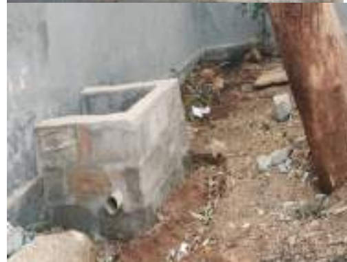
RO Processed water collecting Tank for irrigating the garden
